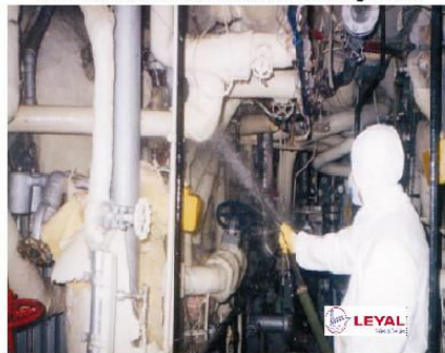
Asbestos removal/disposal is performed according to the most strict National and International regulations
